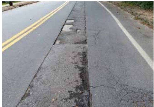
Patchwork done on many neighborhood roads does not comply with the City's Right-of-Way Manual, which requires the entire lane to be resurfaced when cuts are made.
