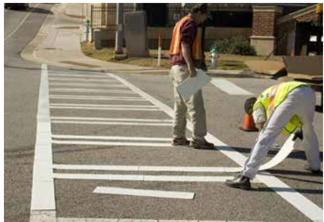
Crosswalks should be repainted where they are worn, substandard, or non-existent.
